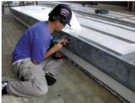
Virginia Tech students got hands-on experience in many phases of building construction. John Rozada attaches C channel at the College of Architecture and Urban Studies Building Research & Demonstration facility.
