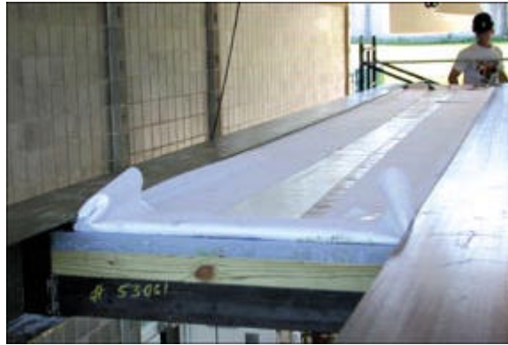
The Acrylife membrane has been attached to the Thermasteel panel and is being wrapped under and then over the fiberglass I-beam. Below: The Thermasteel SIP floor system is inserted between the fiberglass I-beams.
